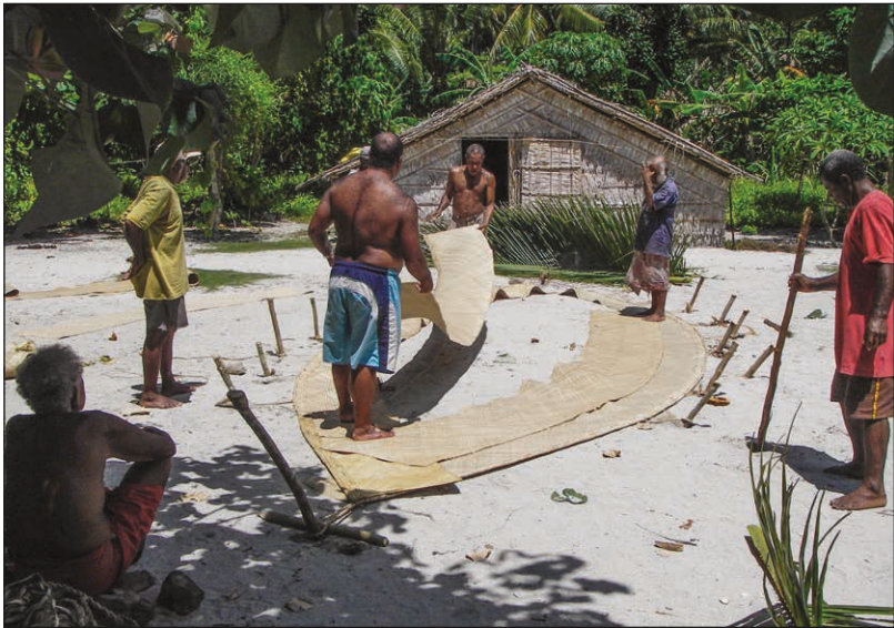
Figure 8. Laying out inner panels after staking of the longest outer panels. Photo by M. George.
